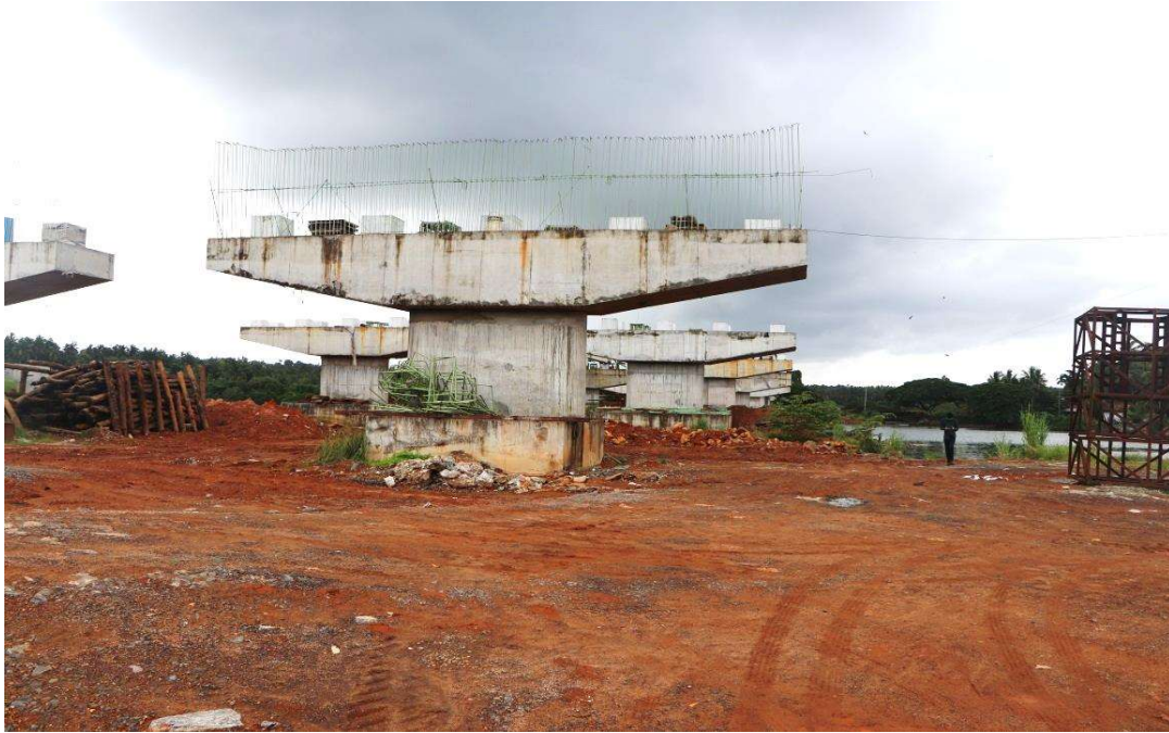
Plate-1: Mangroves removed for Bridge construction at Azhiyur (Location: 75^{\circ}33'2.83''E 11^{\circ}42'11.36''N , Azhiyur Panchayat, Village: Azhiyur)
