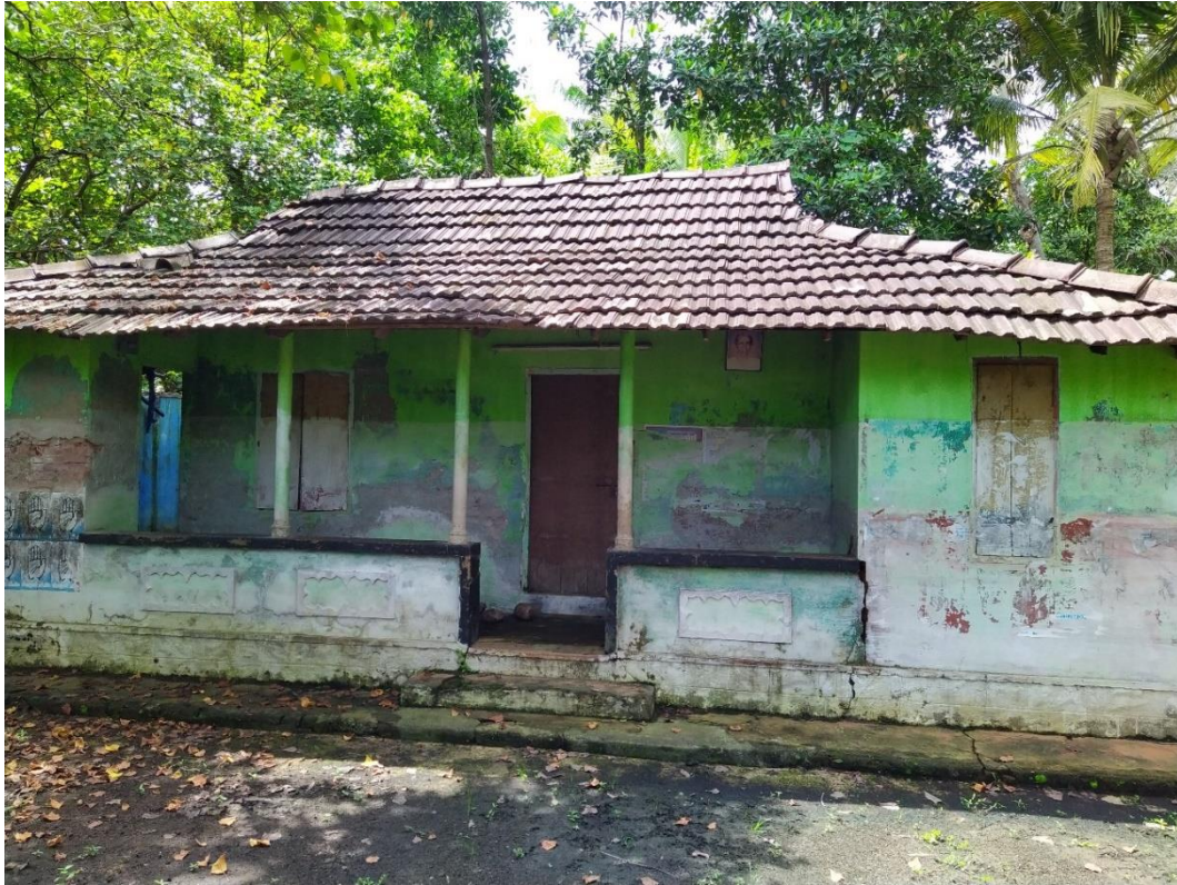
Figure 6: A house in dilapidated condition. Mark of the 2018 flood level can also be seen.
