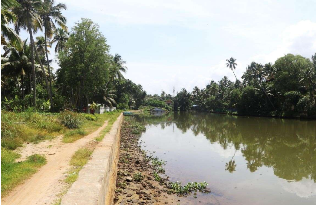
Plate-1: HTL at Embankment construction along the canal at Puthenthura (Location: 76° 32' 4.64" E 8° 58' 6.80" N, Neendakara Panchayat, Village:Neendakara)
