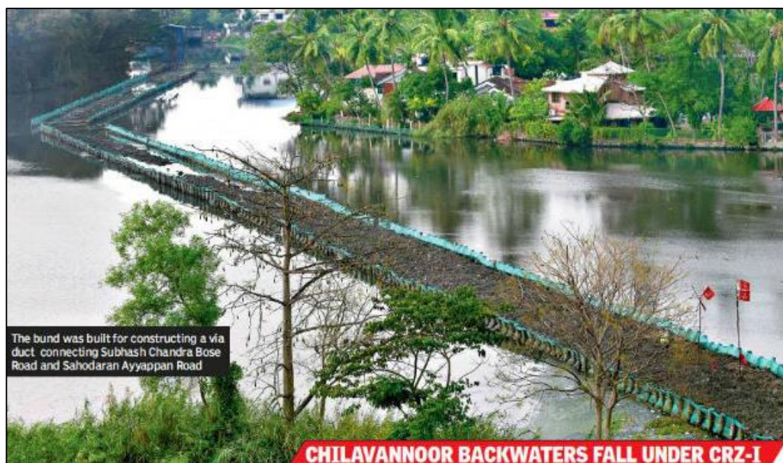
Figure 1: Obstruction of water movement in the Chilavanoor Lagoon within CRZ-I by illegal construction for a walkway not approved by KCZMA
